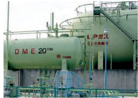
DME貯槽 DME tank
